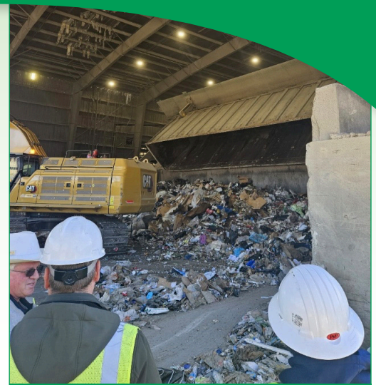
The Authority's James Woods (right) observes as the tipper tilts the rail car and waste falls to the tipping floor.
