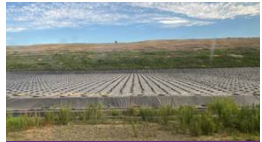
ARM site observation visit of new Phase constructed at ESL for landfilling waste.
